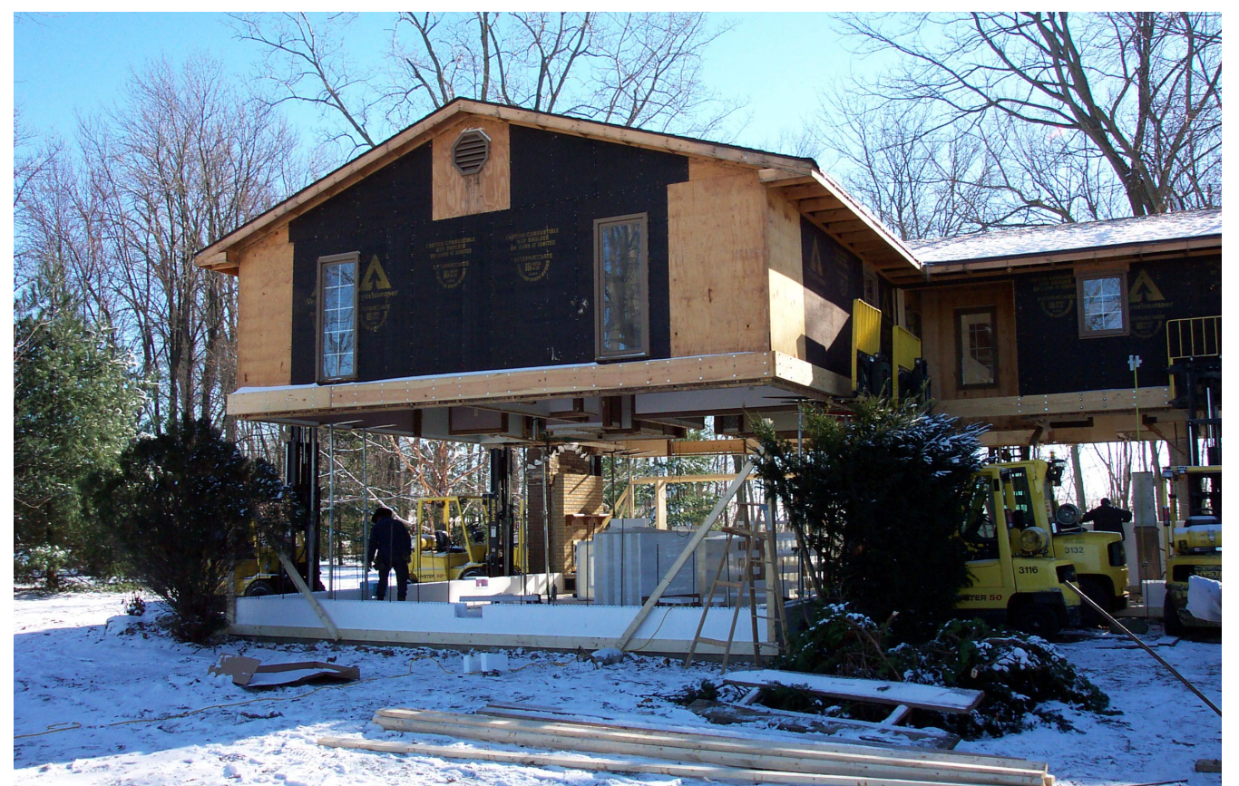
Flood Vents were place within one foot (1’) of the ground. A total of ten (10) Flood Vents were installed to meet FEMA requirements. SMART VENT flood vents were used in this project as they have been approved by FEMA for placement in the walls of enclosed areas. MRBC reserves the right to perform an annual inspection of this home to ensure that vent openings are free of obstruction.
