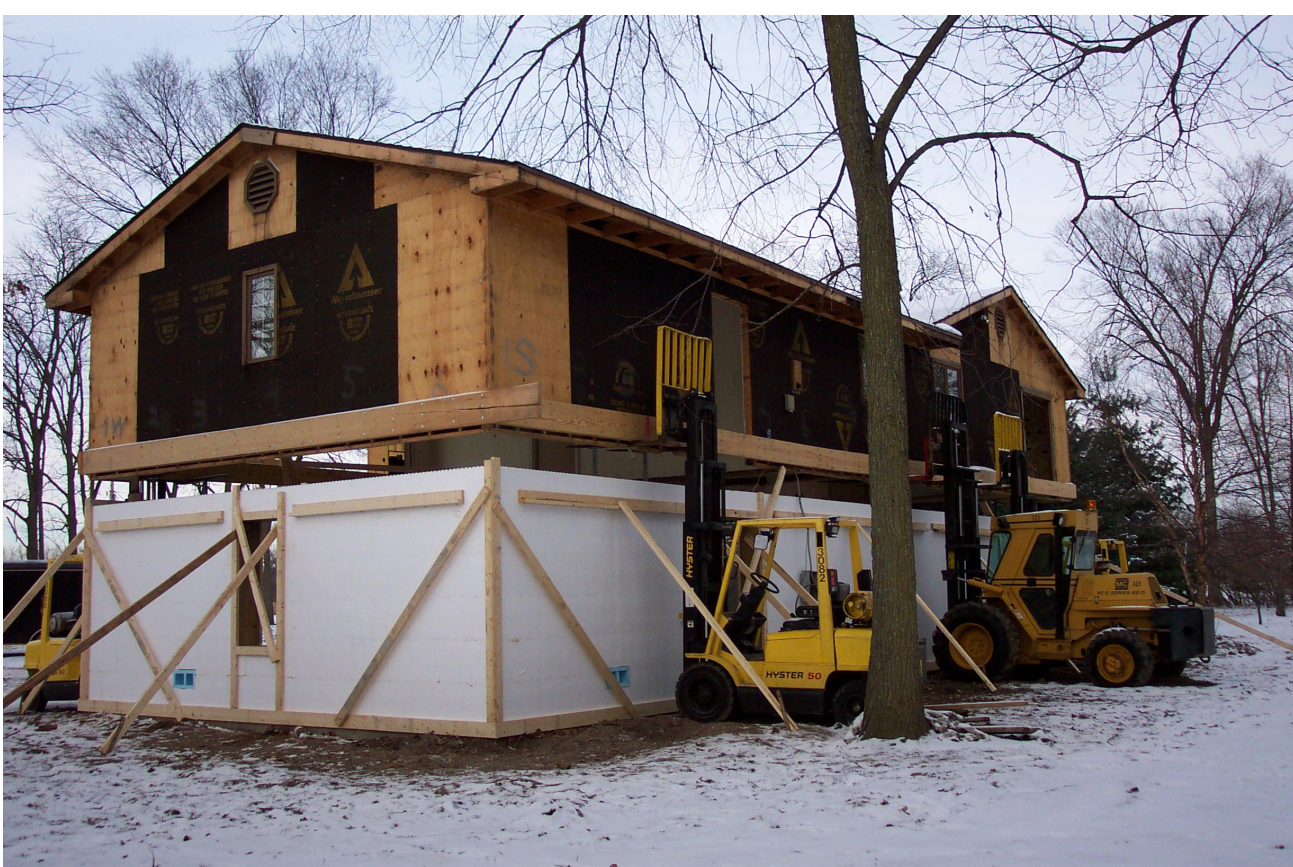
Supporting foundation was constructed using “Insta-form” foundation system blocks. The Styro-foam blocks inter-lock with each other with structural webbing to add strength. Concrete is poured in the forms. Walls have a very high “R” value. Note: “Blue Rectangles” are block-outs for FEMA approved Flood Vents to allow floodwater to flow through the structure.
