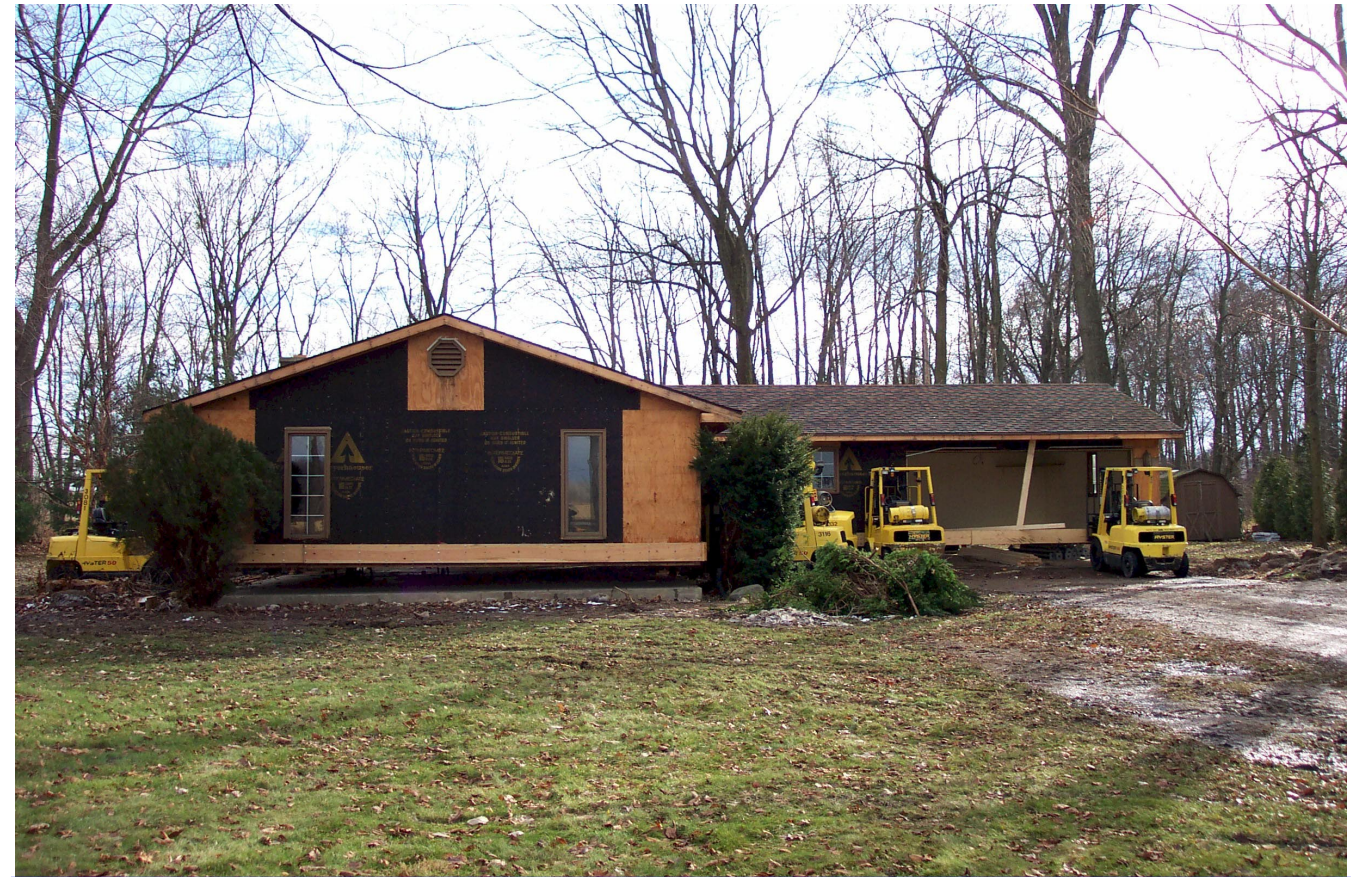
Preparing for “Lift-Off”. A total of ten (10) hydraulic forklifts were used to lift this “slab on grade” structure. Structure’s “L-shaped” configuration contributed to the difficulty in this elevation project.
