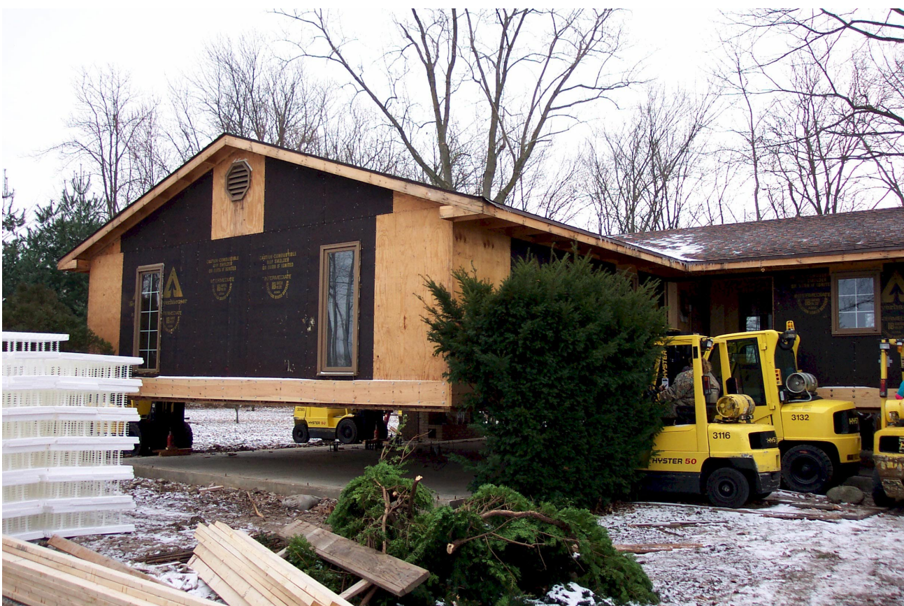
Following examples from the Baton Rouge, Louisiana area, the homeowners chose to lift the structure a total of eight feet (8’). Flood Protection requirements called for elevating the structure +/- five feet (5’). Note: The enclosed area below the structure SHALL NOT be converted to living space per Federal Regulations. Homeowner’s were required to sign a “Deed Restriction”.
